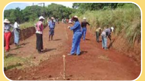
Contractors setting out levels for the labour intensive construction of Nkonjane Road
