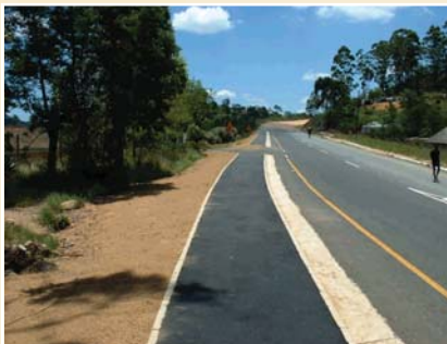
Asphalt sidewalks constructed by Nombuso Lillian Construction (Stage 1) on P68-2, ST Faiths ARRUP project
