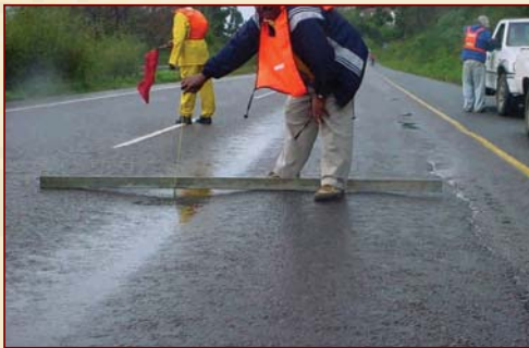
MR82 – August 2002: Serious rutting that is a major roadsafety hazard, especially in wet weather conditions
