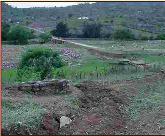
Low level causeway washed away by heavy floods, January 2001
