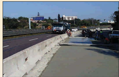
Continuously reinforced concrete layer being layed to a depth of concrete of 240mm to provide for a 30 year service life.
