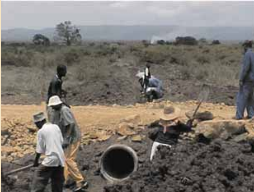
Community workers preparing a drain for headwall at Mkhonjeni Road (Jozini RRTF)
