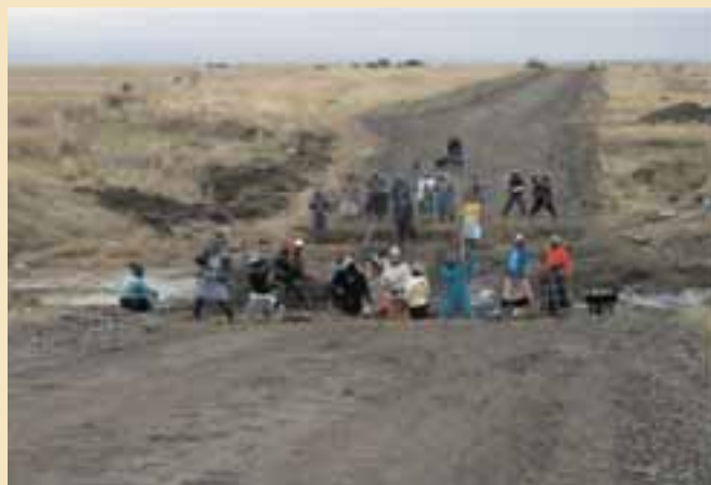
Community workers digging a trench for causeway at Mnxangala Road (Nquthu RRTF)
