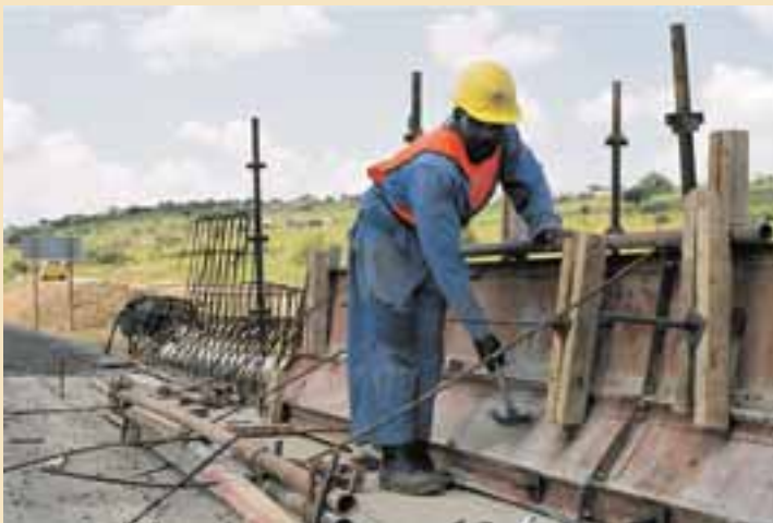
An artisan fitting the concrete shutters on a bridge as a minimum requirement for Site Safety.
