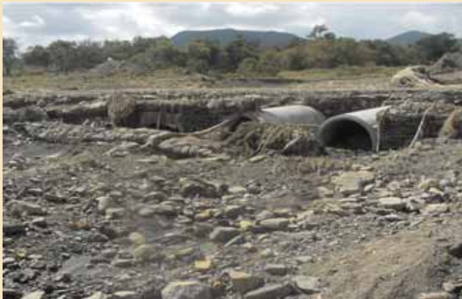
Damaged Mbhekani Structure
