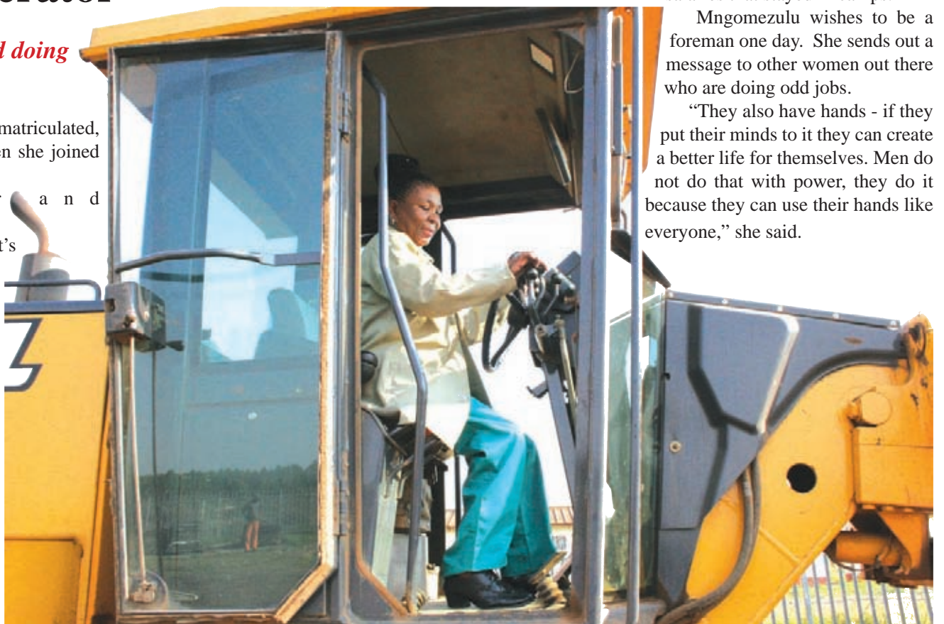
Female grader operator Ms. Sbhongile Mngomezulu of Hluhluwe Cost Centre operates a Departmental grader.
