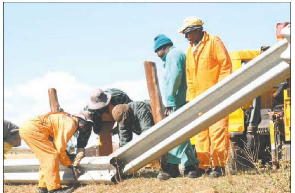
Superintendent Bongani Ngubane supervising Mahlabathini road maintenance team repairing road crash barriers in Mahlabathini.
