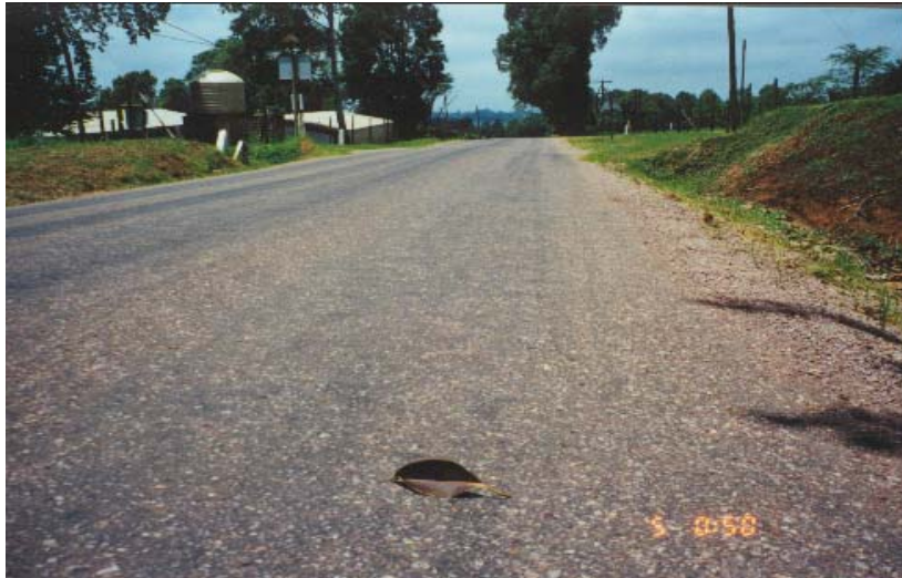
Figure 7: Bleeding along the wheel paths after 6 months.
